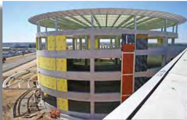
With the roof in place, installation of the terra cotta panels begins on the exterior of the parking ramp entry helix.
